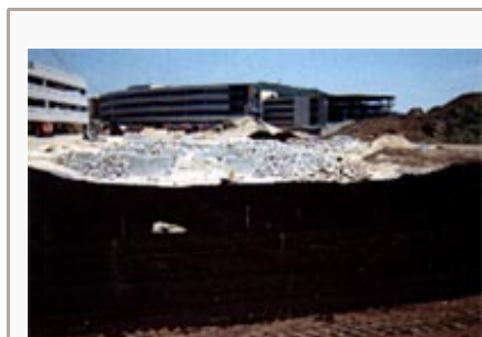
Biologically active compost is used to assure healthy soil and a successful project.
